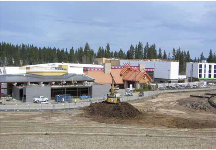
DBS is performing plumbing, electrical and HVAC inspections on this major expansion of the Coeur d'Alene Tribal Casino complex
