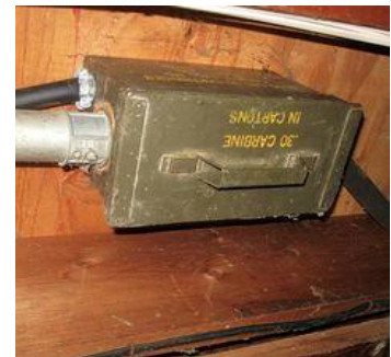
USMC Listed Junction Box
